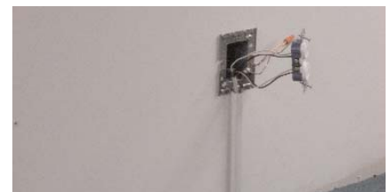
INSTALL SURFACE WIRING BOX PLATE ON EXISTING OUTLET AND WIRE POWER FEED IN FOR ASLL.
